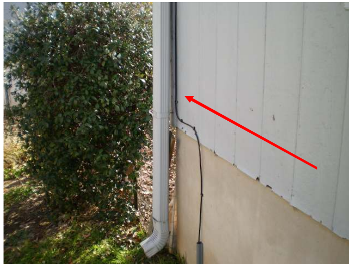
Note: The gutters require cleaning.
