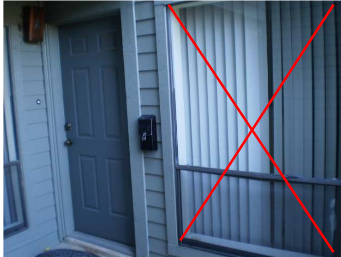
The window sash guide is damaged in the main floor bedroom.
