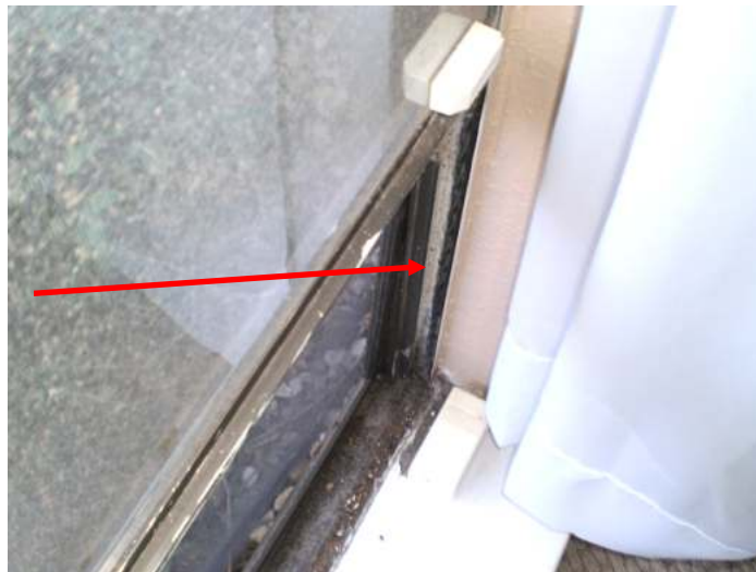
One or more of the windows were observed to be stiff and hard to operate in various locations throughout the house.
