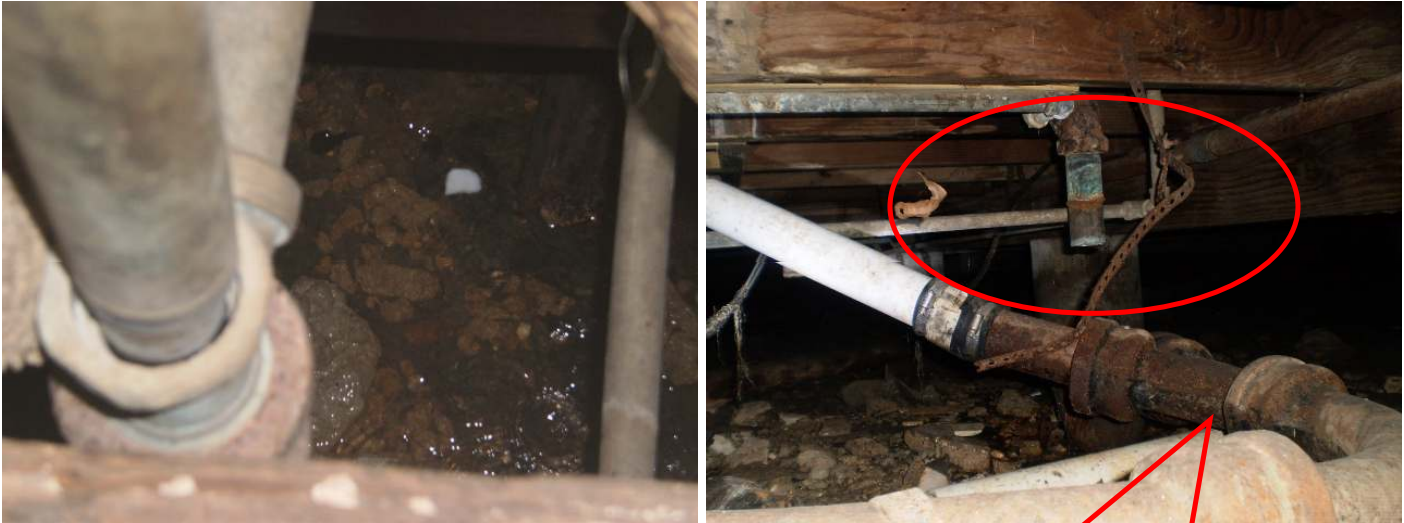
This section of piping has fallen from the support straps; which has pulled loose the drain.
